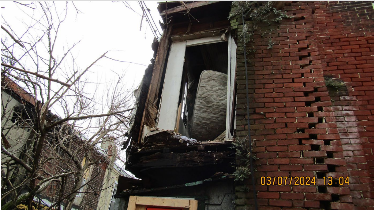
Portions of the ID property have fallen to the ground and sections of loose bricks can weaken the overall structure. It also appears the property sustained fire damage.
