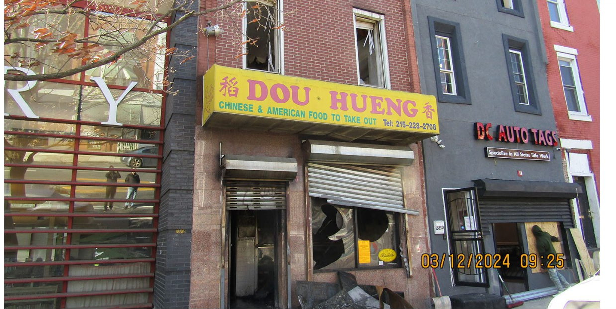
The damage sustained to the commercial ID property created unsecured access points.
