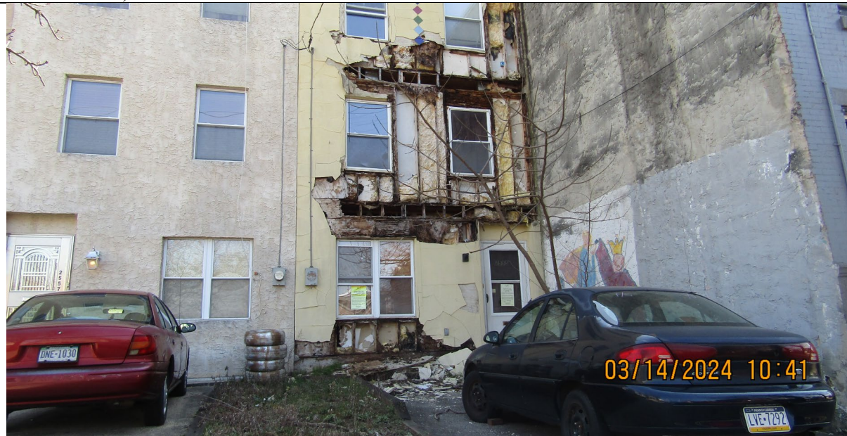
The exterior has sustained significant damage, exposing interior supports.
