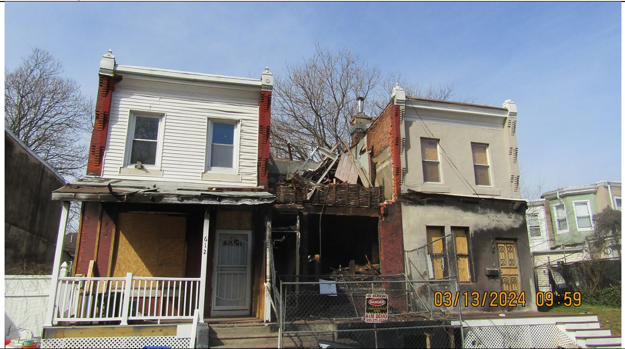
The collapsed middle property created an unsafe environment for the two adjacent structures, which also appear to be unsafe.
