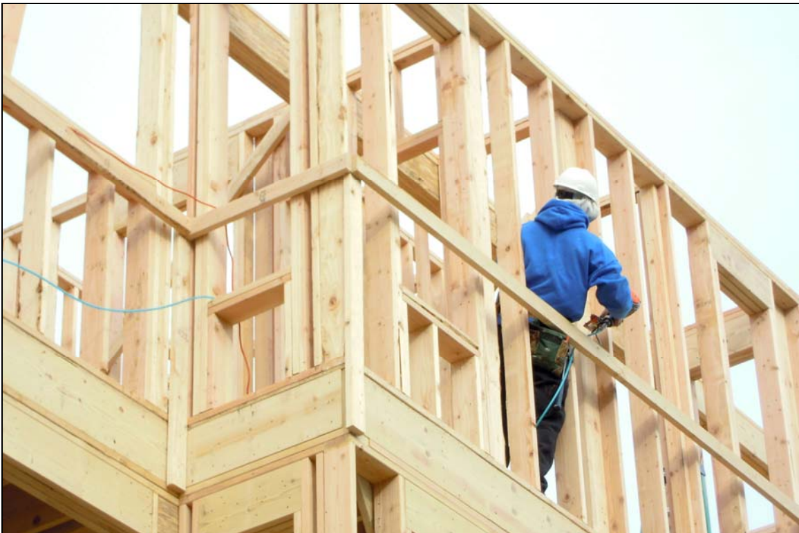
Figure 6 – Worker is not wearing a safety harness. (site 5)
