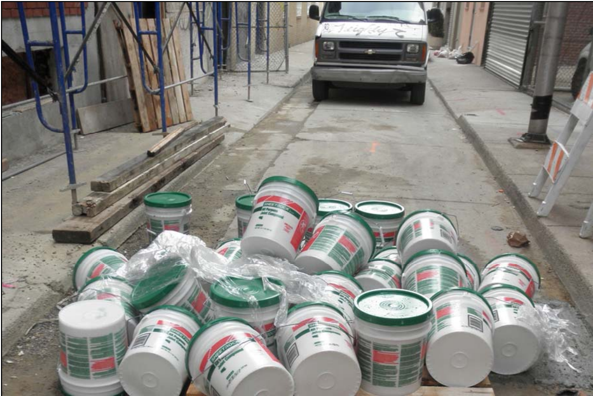
Figure 9 – Pallet of 5 gallon buckets of joint compound toppled into the street blocking traffic (site 2)
