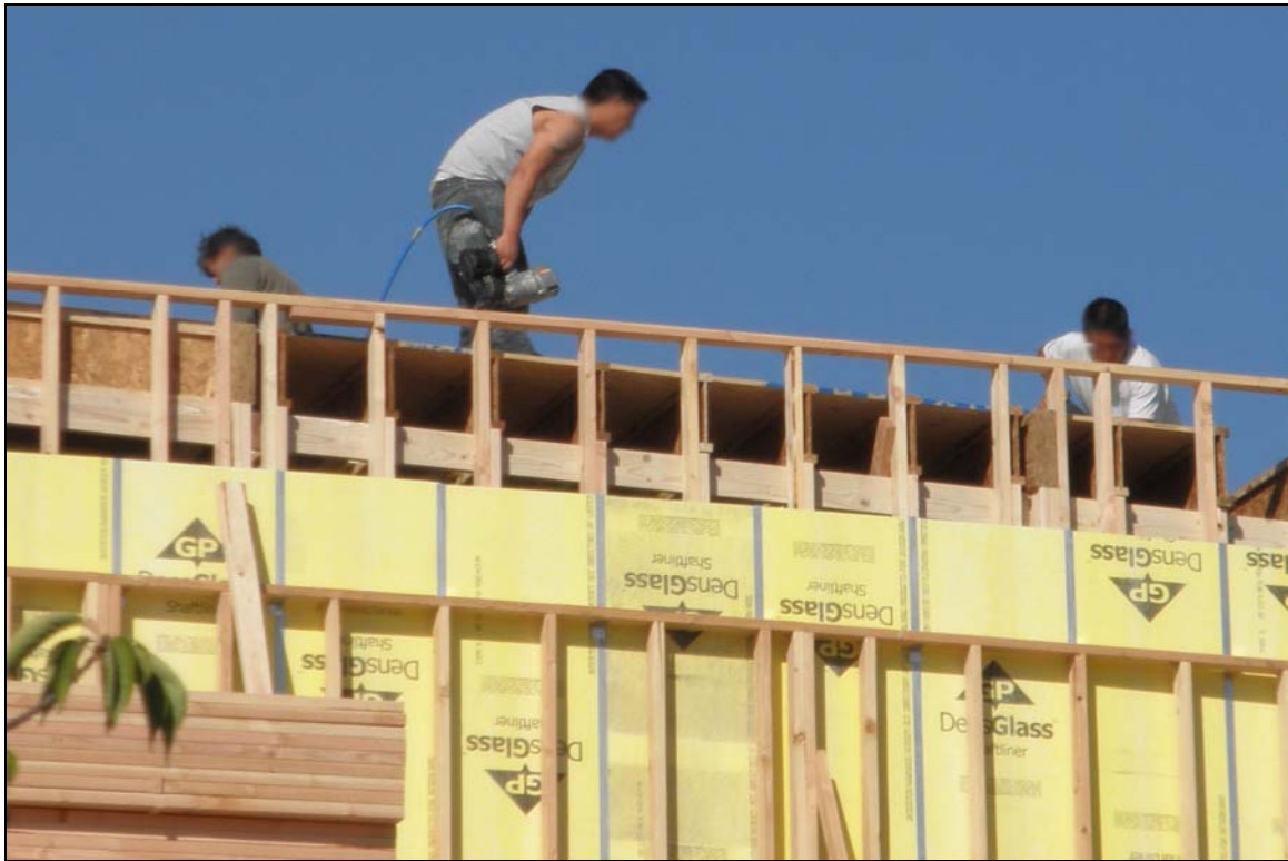
Figure 7 – Workers are not wearing safety harnesses, hard hats or eye protections (site 12)
