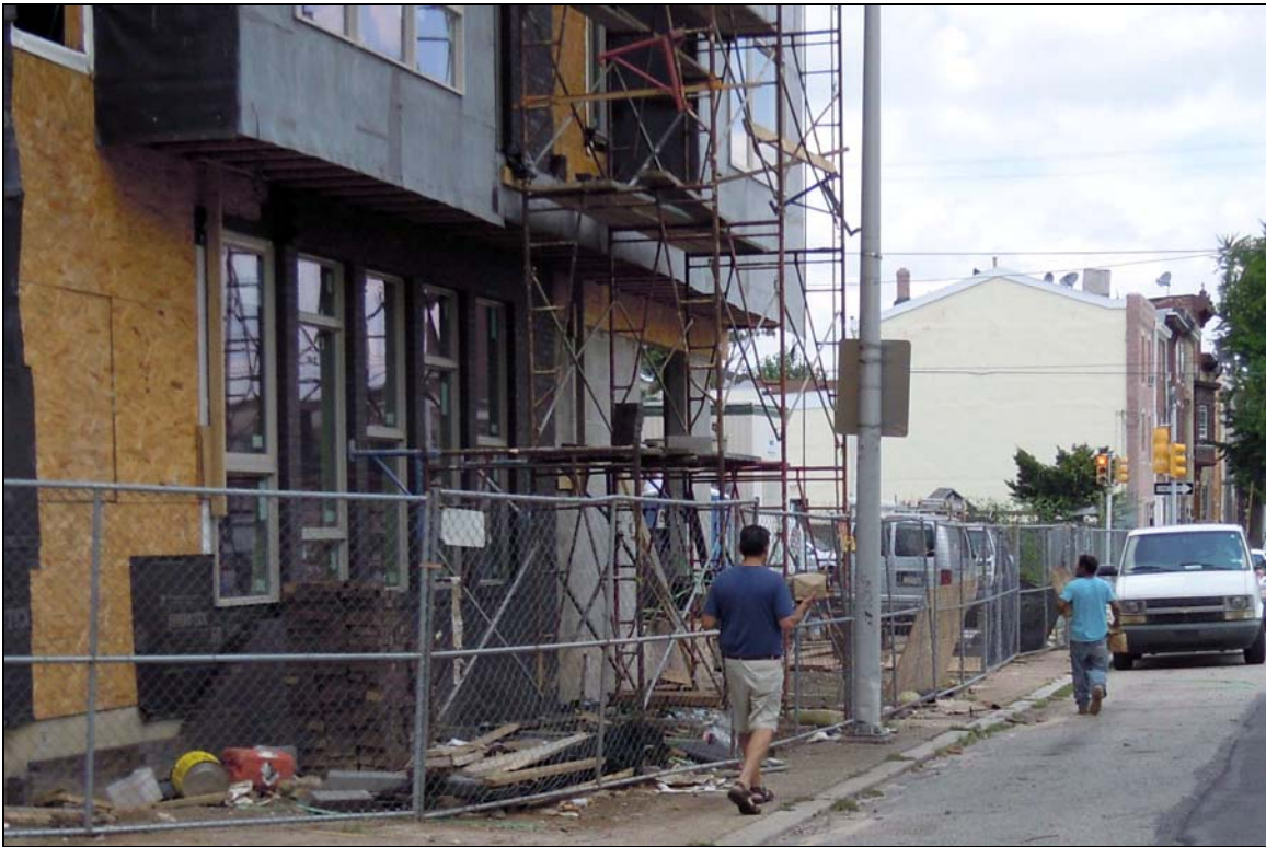
Figure 11 – Unsafe pedestrian conditions. (site 7)
