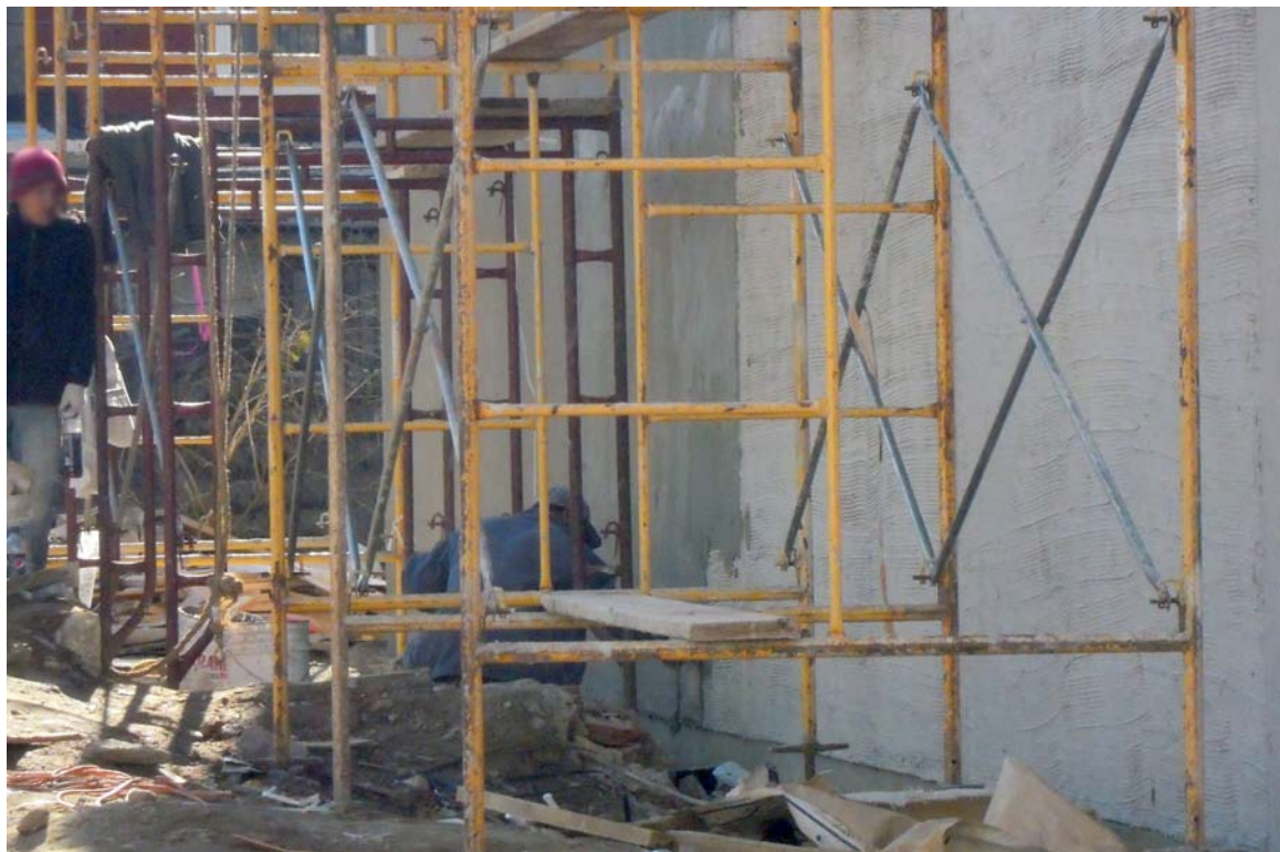
Figure 16 – Scaffolding not properly secured to the wall or the ground. (site 9)
