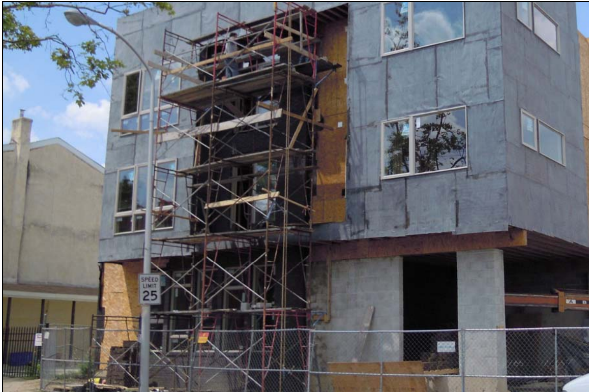
Figure 15 – Scaffolding does not appear secure. (site 7)
