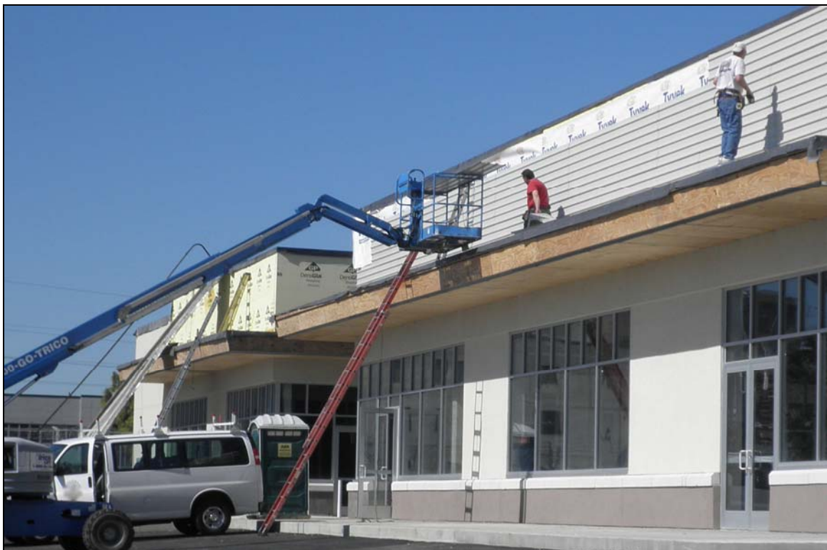
Figure 8 – Workers are not wearing hard hats or safety harnesses. (site 18)
