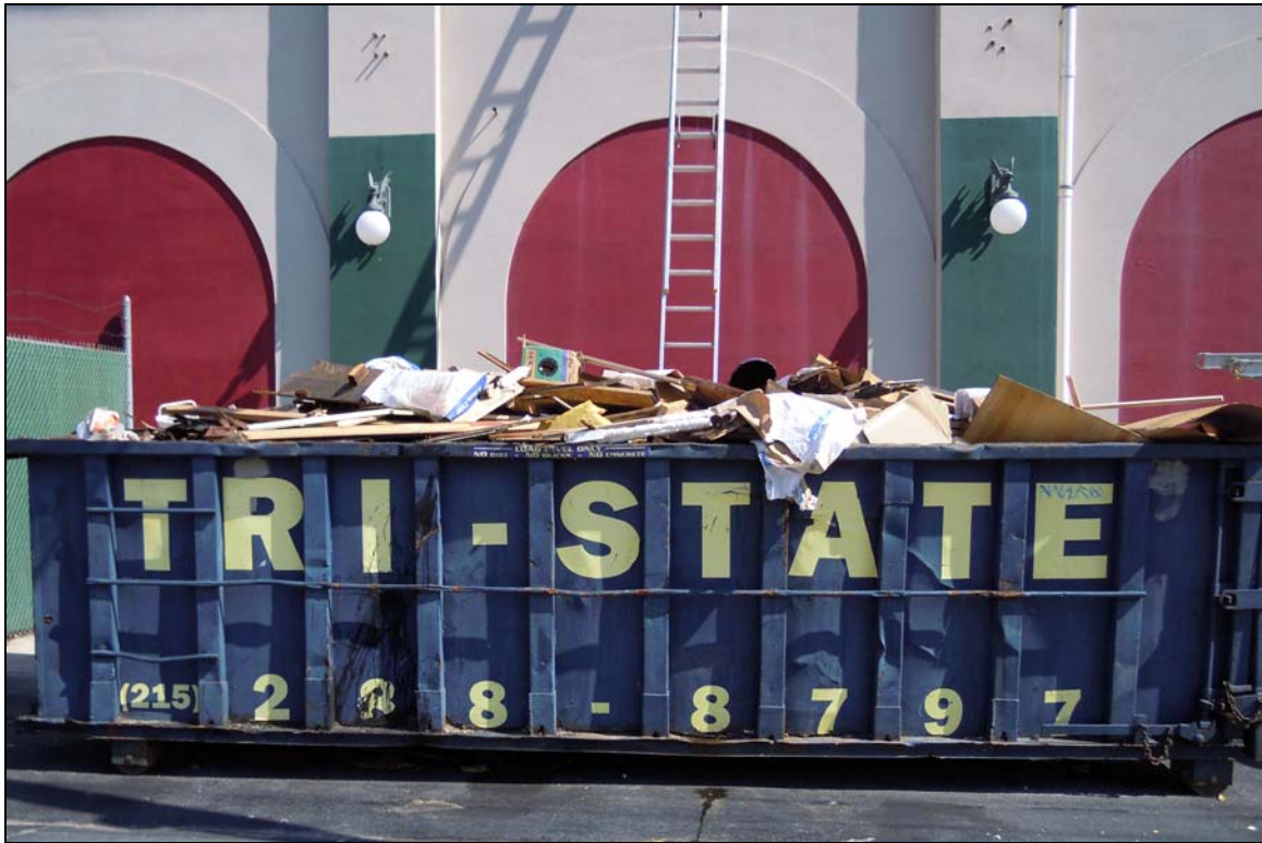
Figure 13 – Dumpster surpassed capacity. (site 15)
