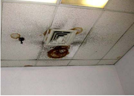
Figure 13 – Air Ducts need to be cleaned: Carousel House
