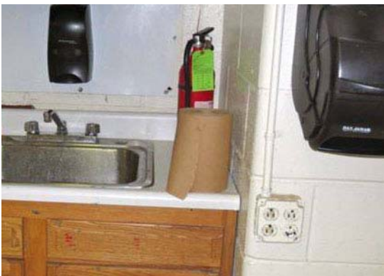
Figure 29 - Outlet should have GFCI: Heitzman
