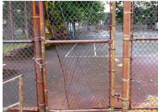
Figure 52 – Damaged Fence: Morris Estate
