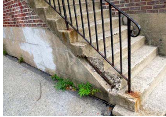
Figure 32 – Damaged Masonry: Kendrick
