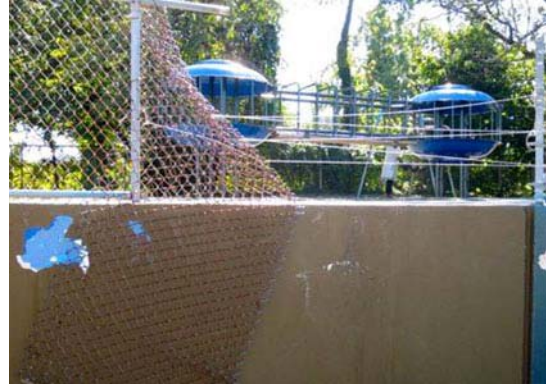
Figure 50 – Damaged Fence: McCreech
