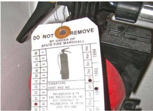
Figure 45 – Expired Fire Extinguisher: Mantua
