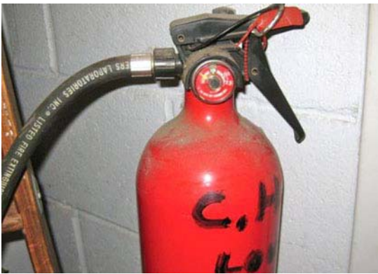
Figure 9 – Fire Extinguisher empty with no tag: Carousel House
