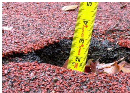
Figure 54 – Damaged Safety Surface: Morris Estate
