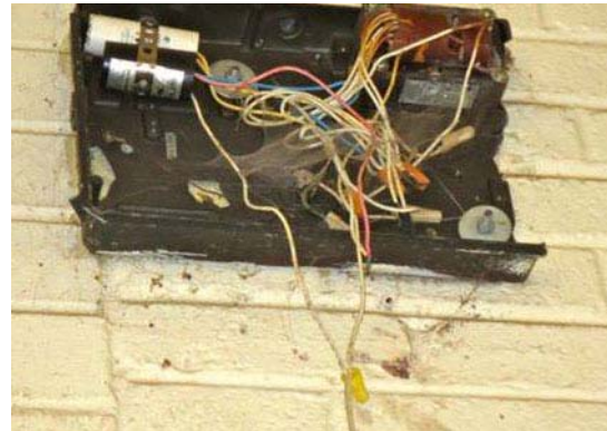
Figure 64 – Exposed Wires: Papa
