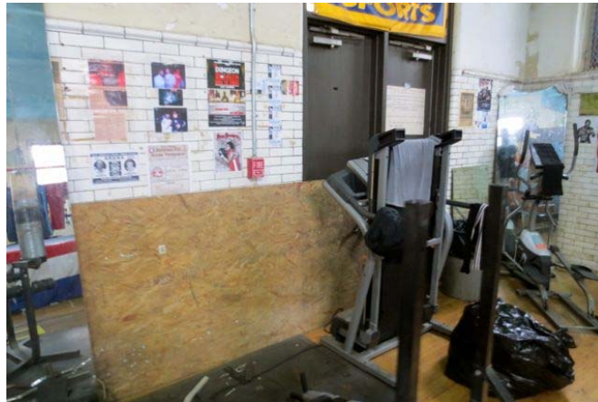
Blocked Fire Exit: Athletic
