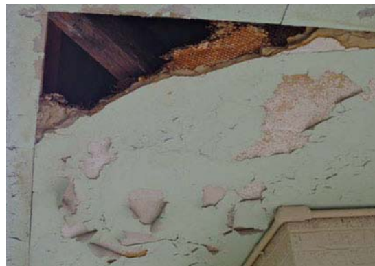
Figure 30 - Deteriorated Side Fascia: Jacobs
