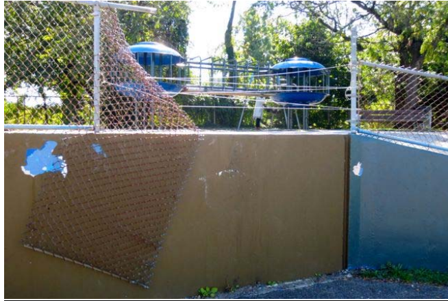
Damaged Fence: McCreesh
