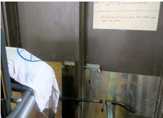
Figure 5 – Blocked Fire Exit: Athletic
