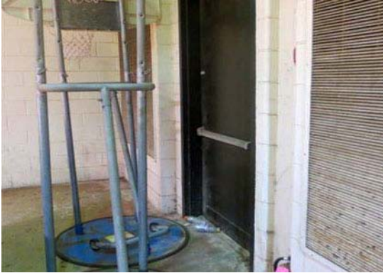
Figure 61 – Blocked Fire Exit: Palumbo
