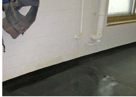
Figure 14 – Water Leaking in Building: Carousel House
