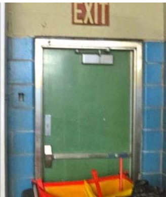
Figure 75 – Blocked Fire Exit: Schmidt
