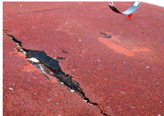
Figure 84 - Damaged Safety Surface: Ziehler
