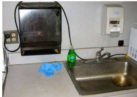
Figure 12 –Outlet should have GFCI: Carousel House
