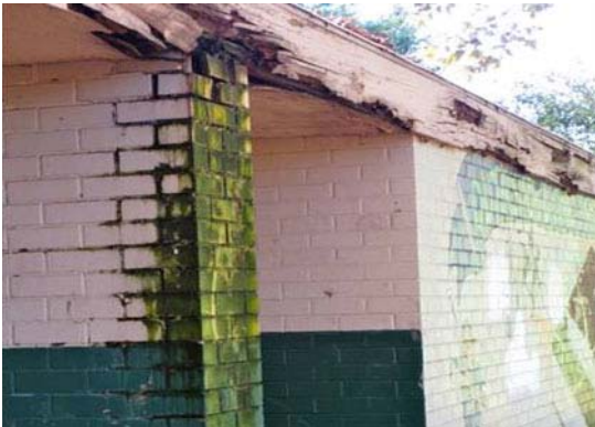
Figure 63 – Damaged Roof and Gutter: Papa
