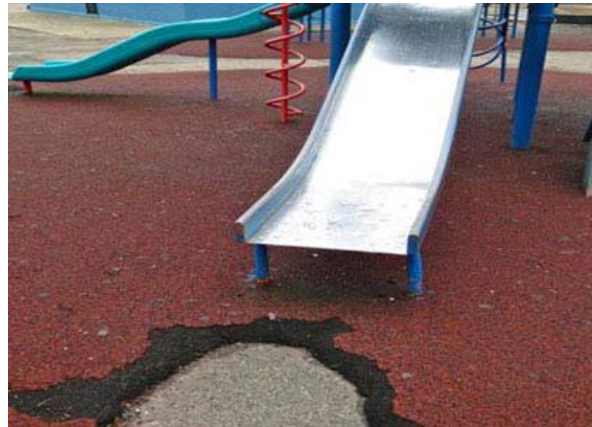
Damaged Safety Surface: Stokley
