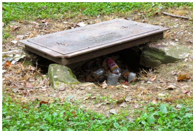
Tripping Hazard: Morris Estate
