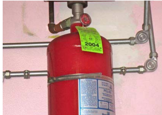
Figure 58 – Expired Fire Extinguisher: Morris Estate
