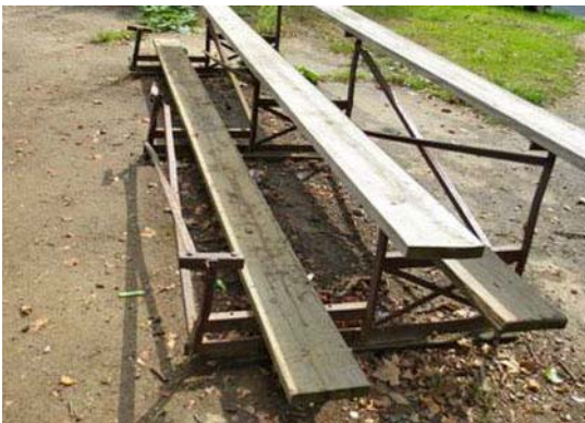
Figure 41 – Damaged Bleachers: Lee
