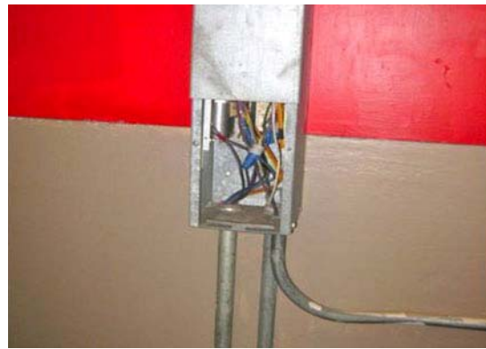
Figure 46 – Exposed Wires: Mantua
