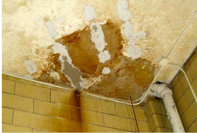
Water Damage: Lawncrest
