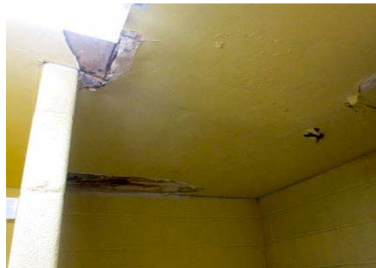
Figure 76 – Damaged Ceiling: Schmidt
