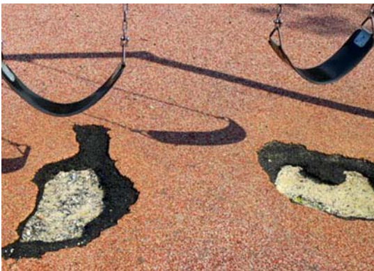
Figure 39 – Damaged Safety Surface: Lawncrest
