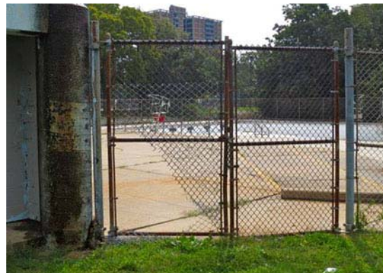
Figure 42 – Damaged Fence: Lee
