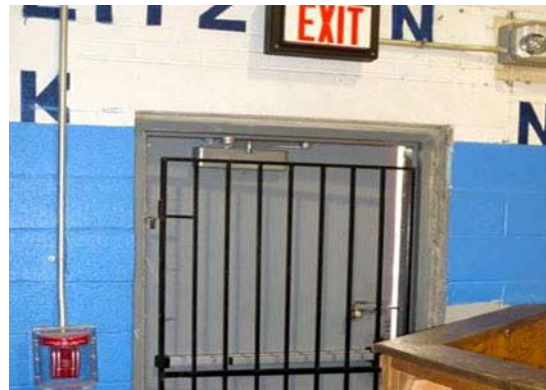
Figure 28 - Locked Fire Exit: Heitzman
