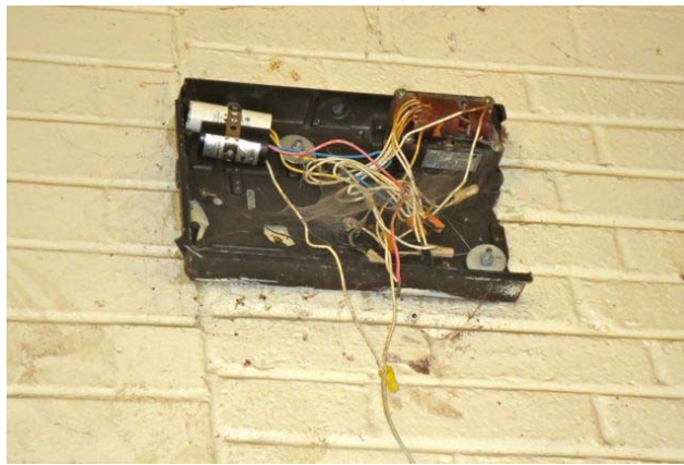
Exposed Wires: Papa
