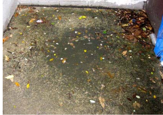
Figure 44 – Clogged Drain: Mantua
