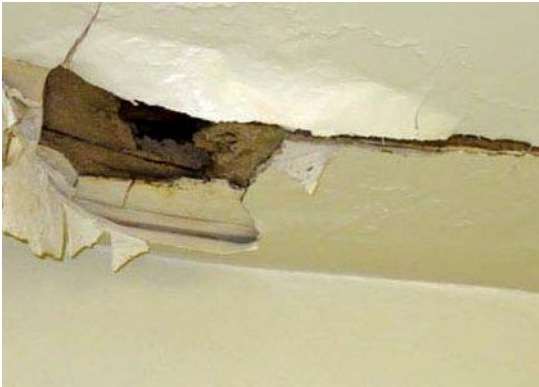
Figure 57 – Damaged Ceiling: Morris Estate
