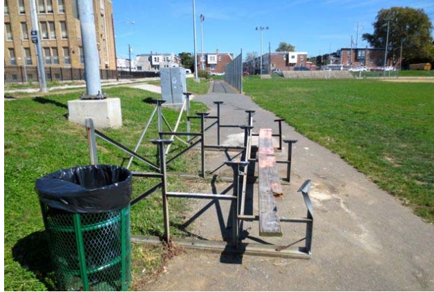
Damaged Bleacher: McCreesh
