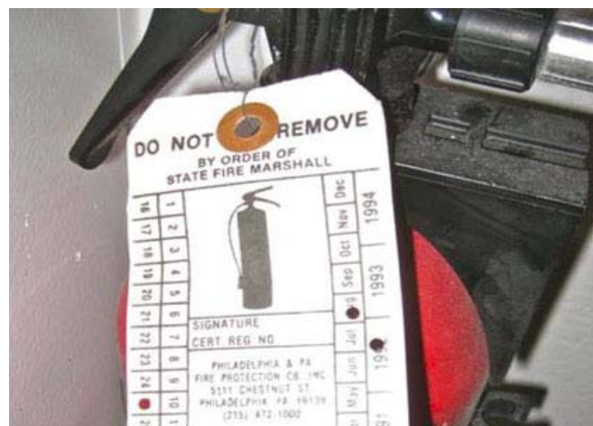
Expired Fire Extinguisher: Mantua
