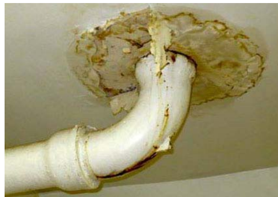
Figure 60 – Water Damage: Morris Estate
