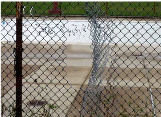
Figure 27 - Damaged Fence: Heitzman
