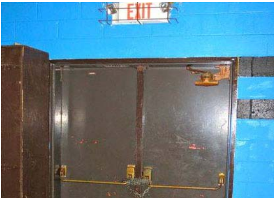
Figure 15 – Fire Exit Locked: Christy
