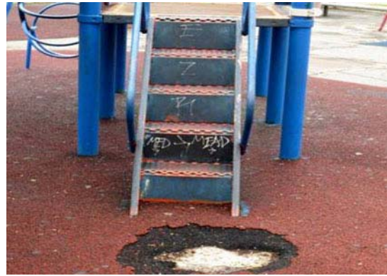
Figure 80 – Damaged Safety Surface: Stokley
