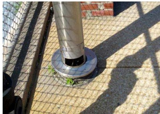
Figure 78 – Exposed Wires: Schmidt
