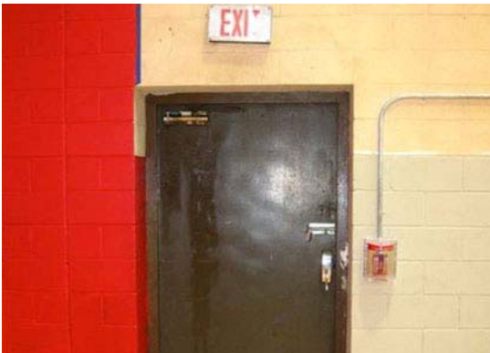
Figure 47 – Locked Fire Exit: Mantua
