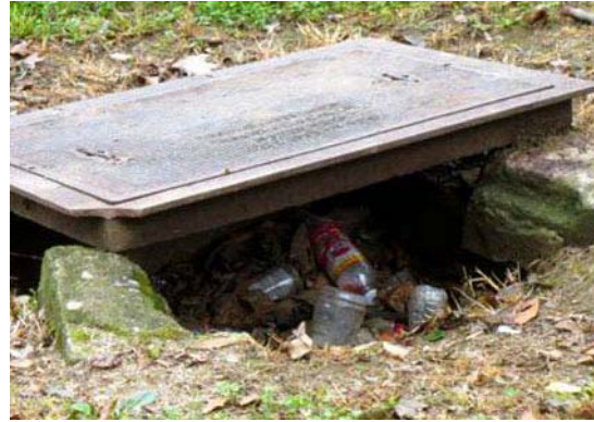
Figure 56 – Tripping Hazard: Morris Estate
