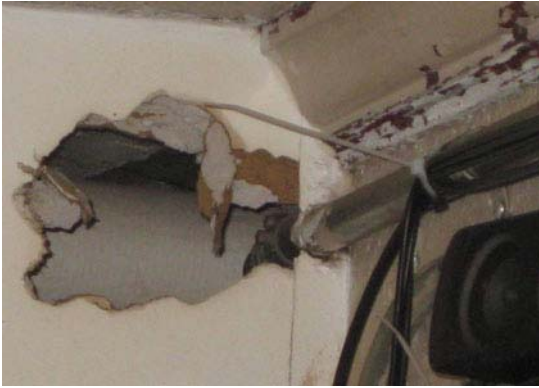
Figure 73 – Hole in Wall: Sacks
