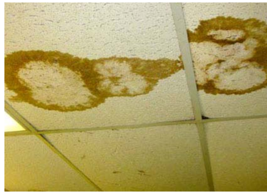
Figure 10 – Leaking Ceiling: Carousel House
