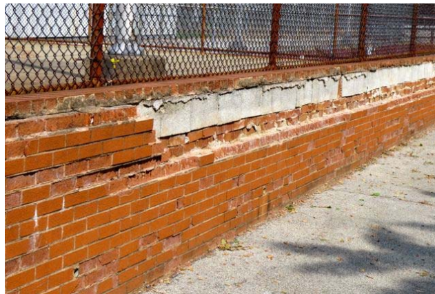
Damaged Masonry Wall: Lawncrest
