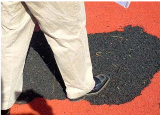
Figure 77 – Damaged Safety Surface: Schmidt
