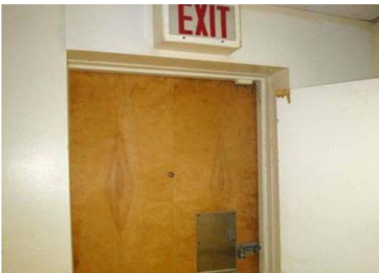
Figure 59 – Locked Fire Escape: Morris Estate
