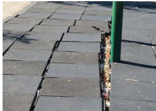
Figure 16 – Safety Surface Damaged: Columbus
