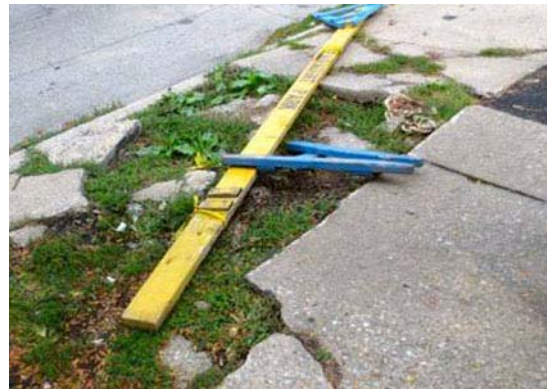
Figure 22 – Damaged Sidewalk: Cruz
