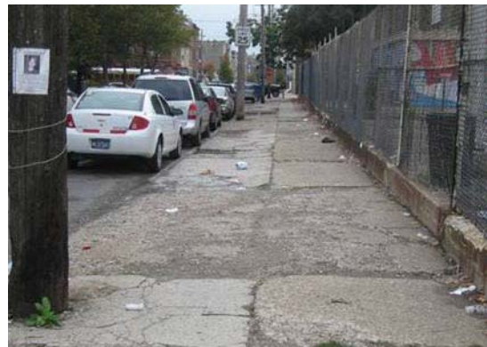
Figure 72 - Damaged Sidewalk: Sacks
