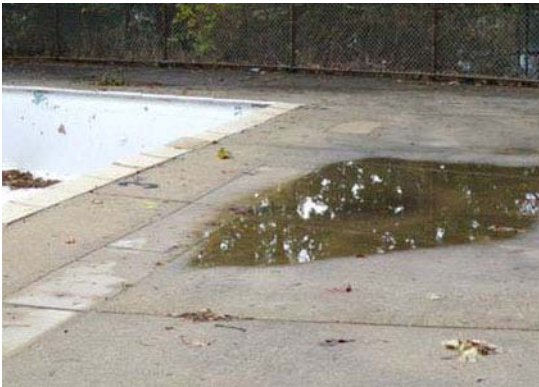
Figure 51 – Clogged Drain: Morris Estate
