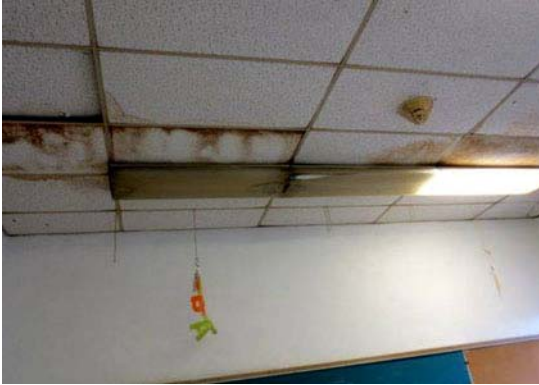
Figure 7 – Water Damage: Athletic
