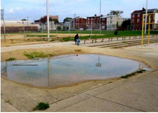
Figure 25 - Clogged Storm Drain: Cruz
