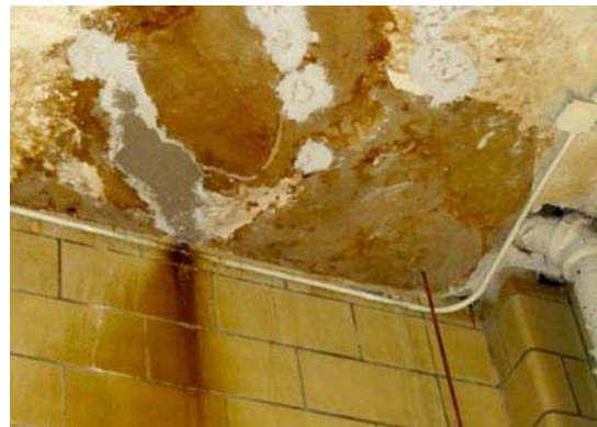
Figure 40 – Water Damage: Lawncrest
