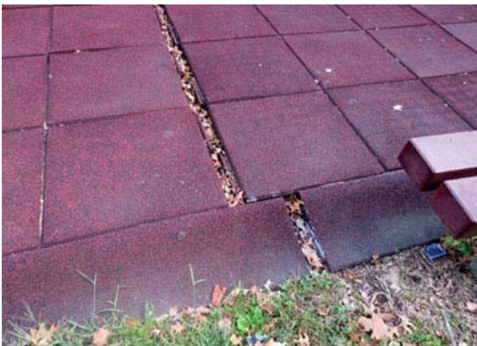
Figure 71 - Gap in Safety Surface: Mallery
