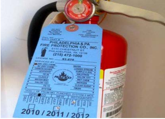
Figure 19 – Expired Fire Extinguisher: Columbus
