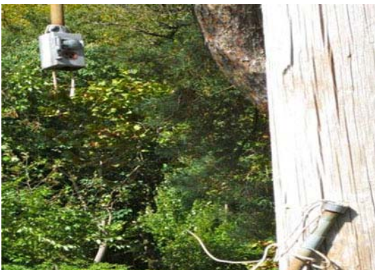
Figure 65 – Exposed Wires: Papa
