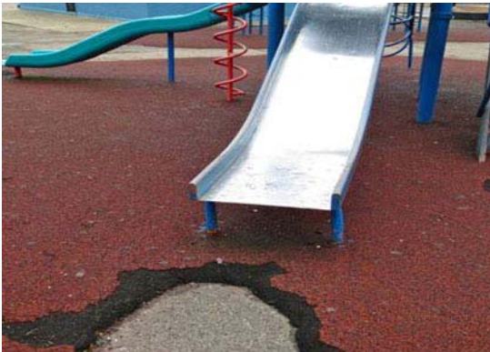
Figure 81 – Damaged Safety Surface: Stokley
