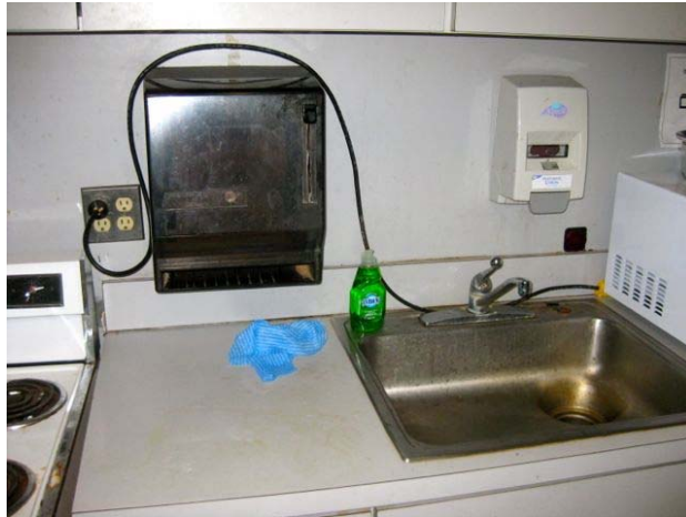
Outlet should have GFCI: Carousel House
