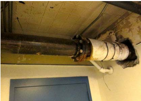
Figure 33 – Exposed Hot Pipe Drips: Kendrick
