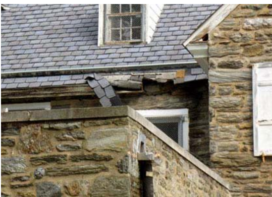
Figure 53 – Damaged Roof and Gutters: Morris Estate
