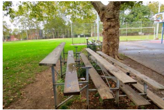
Figure 4 – Damaged Bleachers: Athletic
