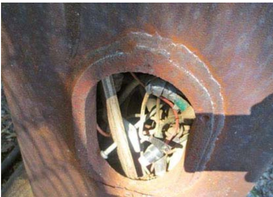
Figure 17 – Exposed Wires: Columbus
