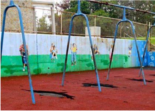
Figure 55 – Missing Swings and Damaged Safety Surface: Morris Estate
