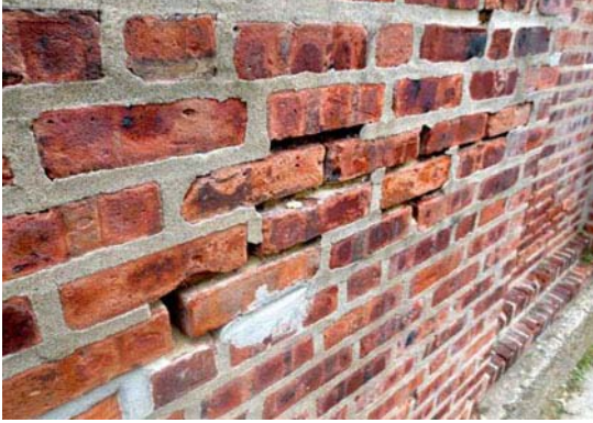
Figure 31 – Pool Wall needs Mortar: Kendrick
