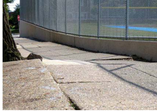
Figure 68 - Tripping Hazard: Ramp
