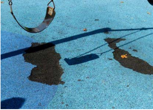
Figure 67 - Damaged Safety Surface: Ramp
