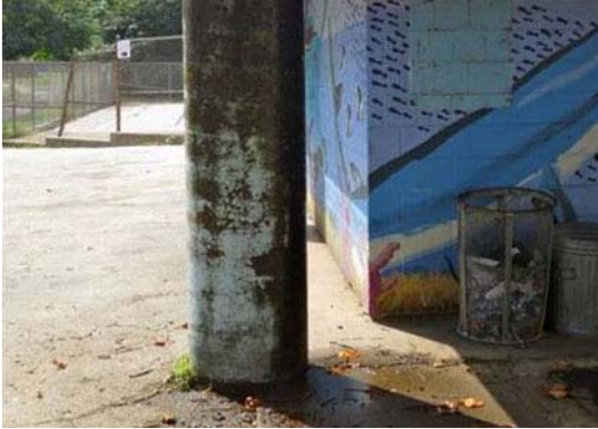
Figure 43 – Leaking Gutters: Lee
