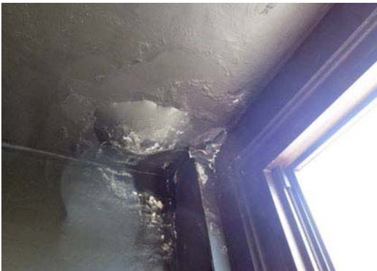
Figure 35 – Water Damage: Kendrick
