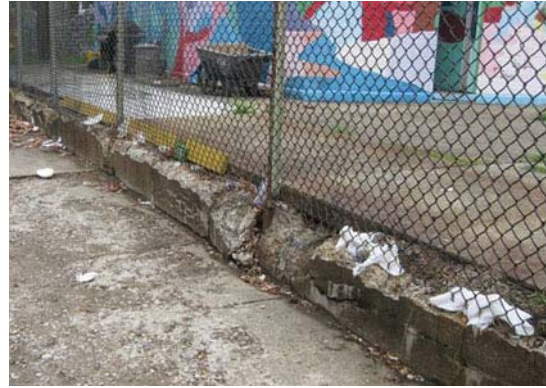
Figure 74 – Damaged Sidwalk: Sacks
