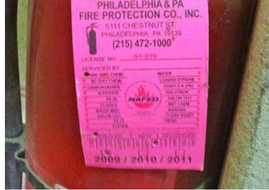
Figure 62 – Expired Fire Extinguisher: Palumbo
