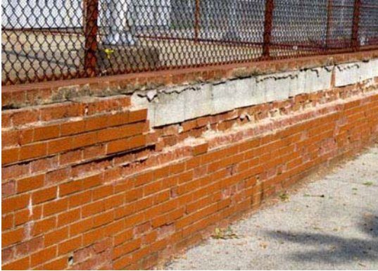
Figure 37 – Damaged Masonry Wall: Lawncrest
