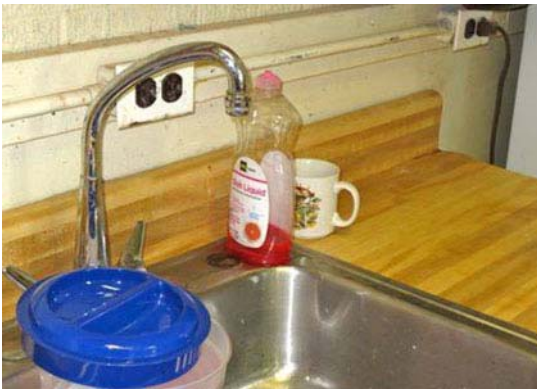
Figure 69 - Outlet should have GFCI: Roosevelt
