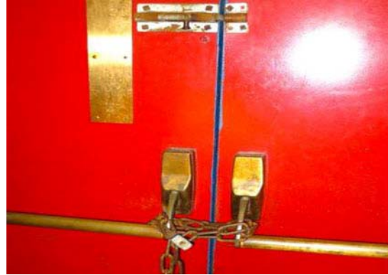
Figure 38 – Locked Fire Exit: Lawncrest
