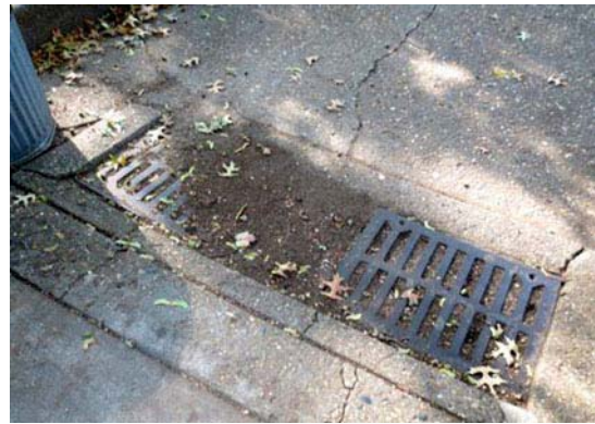
Figure 70 - Clogged Drain: Mallery
